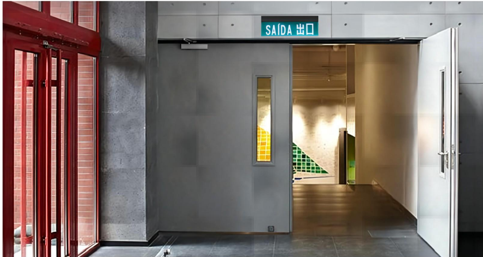
Passage Corridor Fire-Rate Door
